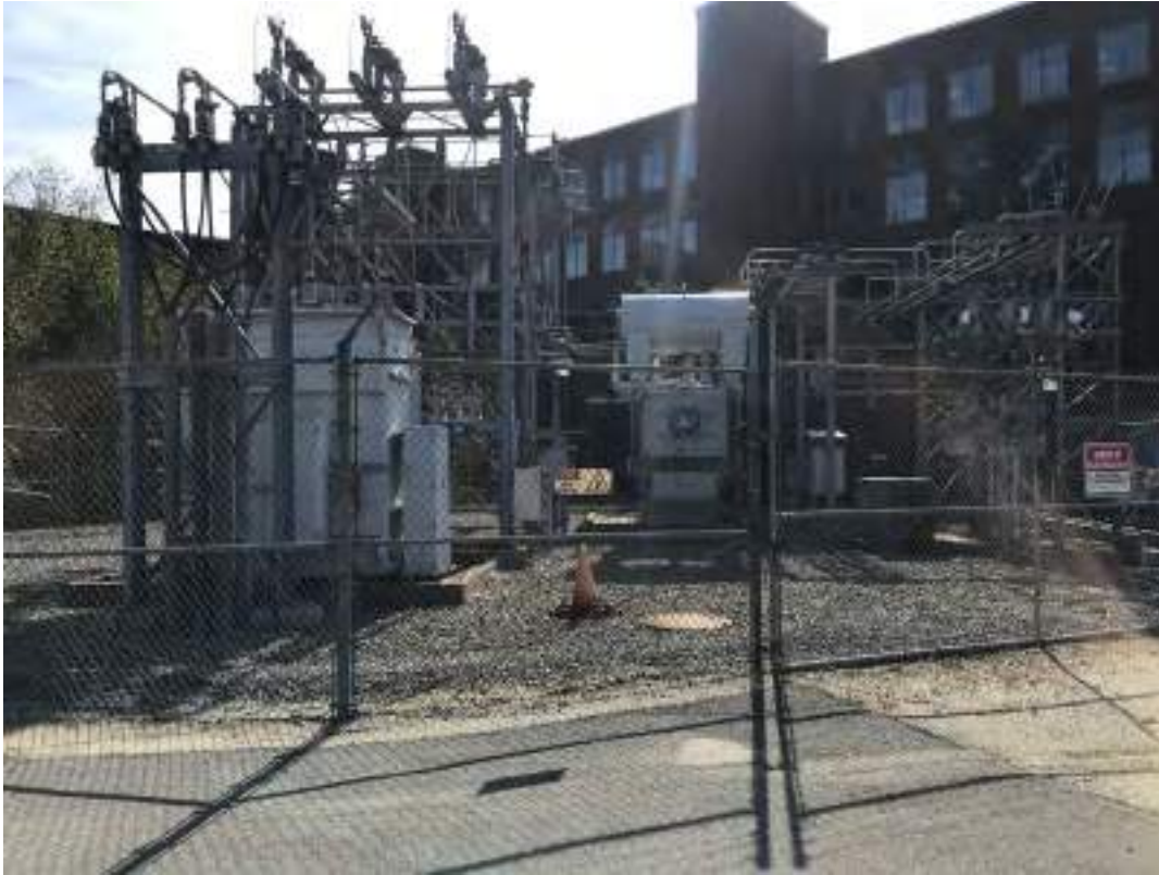
Photo 3-8: Project Interconnection Point
